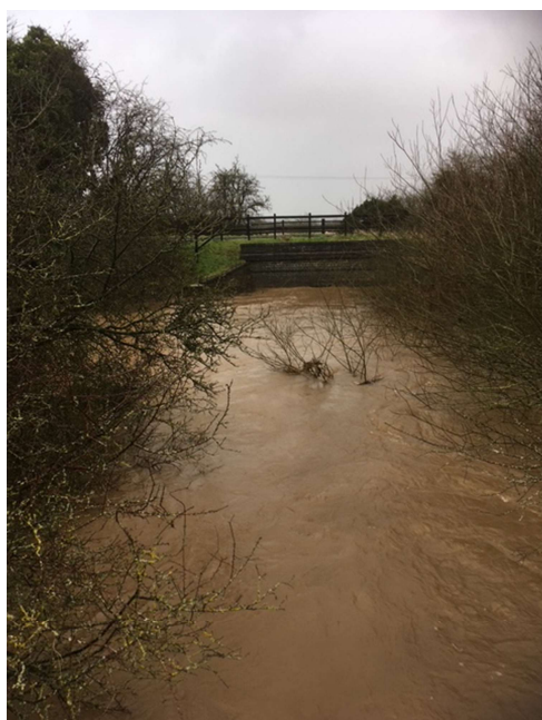
Figure 2.4: Canal aqueduct 21 Feb 2022 flood water over arch level
