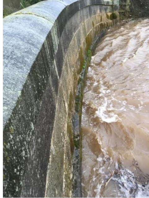
Figure 2.5: Monks Bridge Complex showing 21 Feb 2022 flood water up to top of arch
